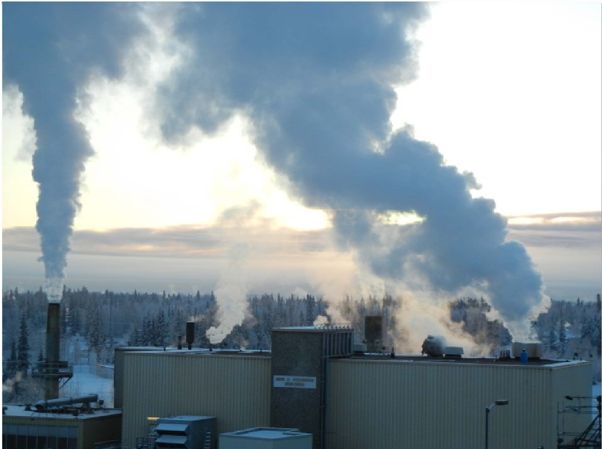
Emissions from UAF coal-fired power plant
