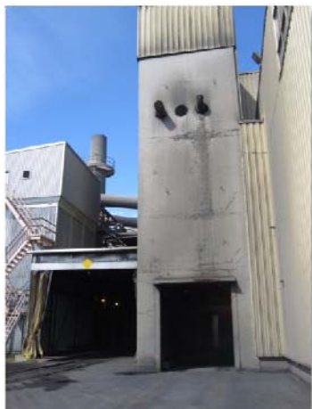
UAF coal ash loading bay
