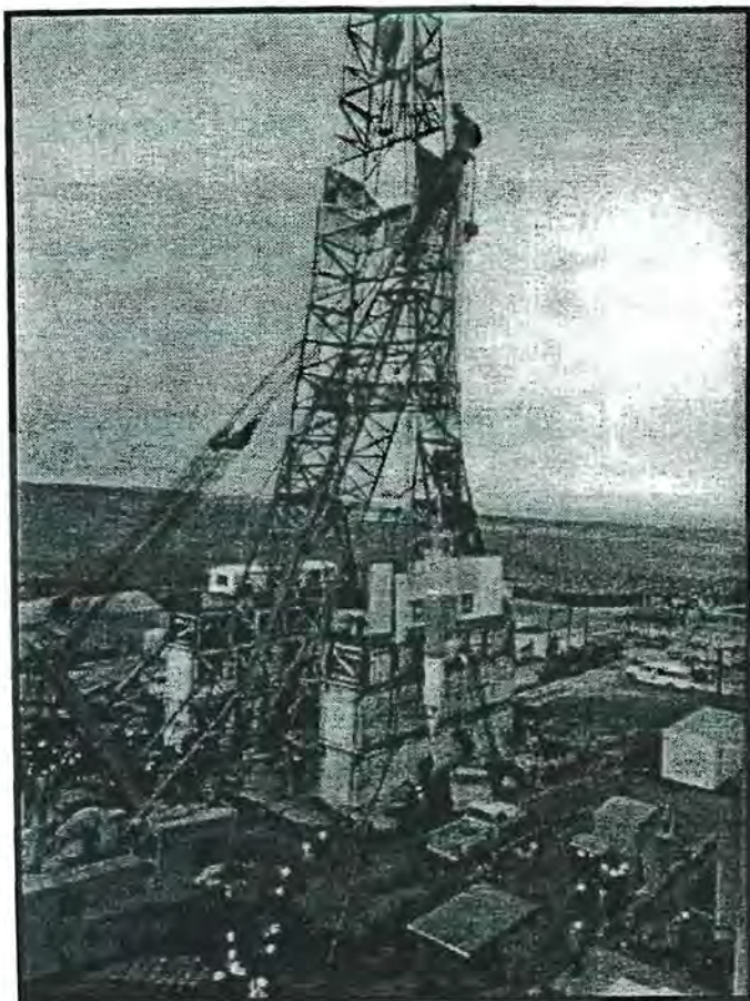
Photo courtesy U.S. Department of Energy
