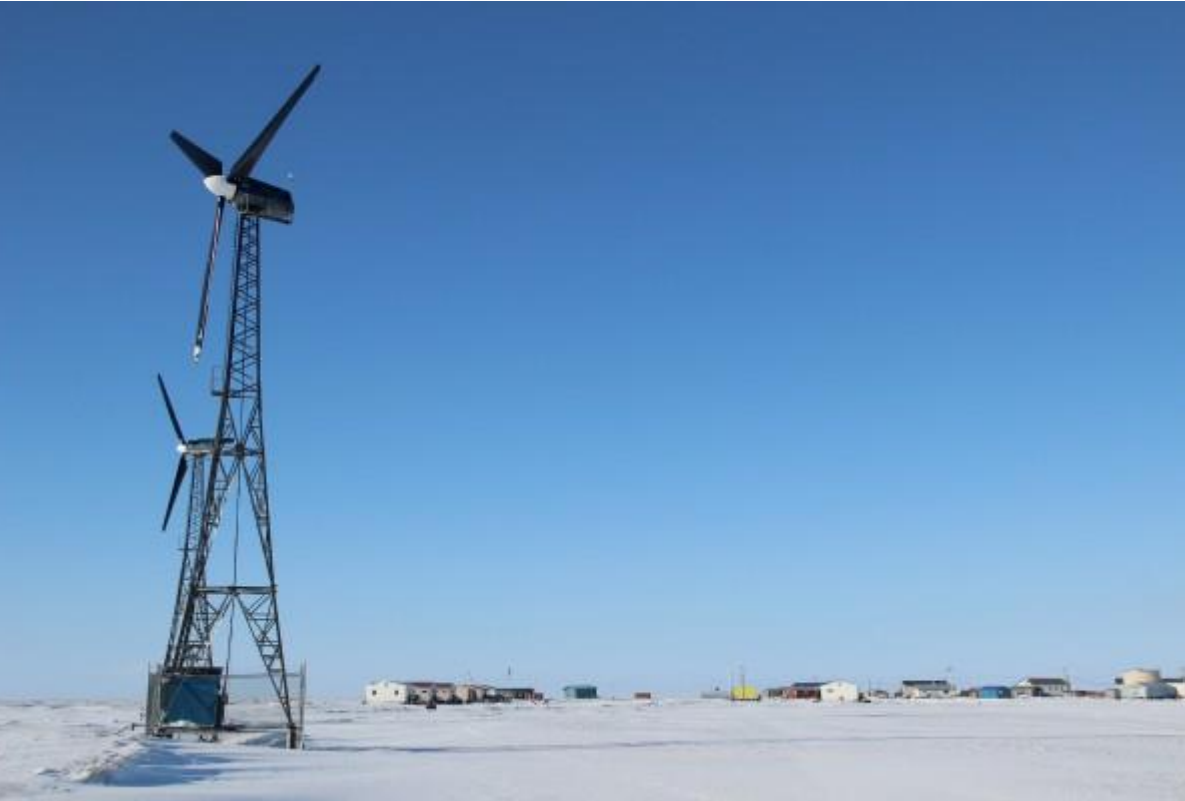
Kwigillingok has five wind turbines, four of which are currently working. Photo: Rachel Waldholz/APRN
