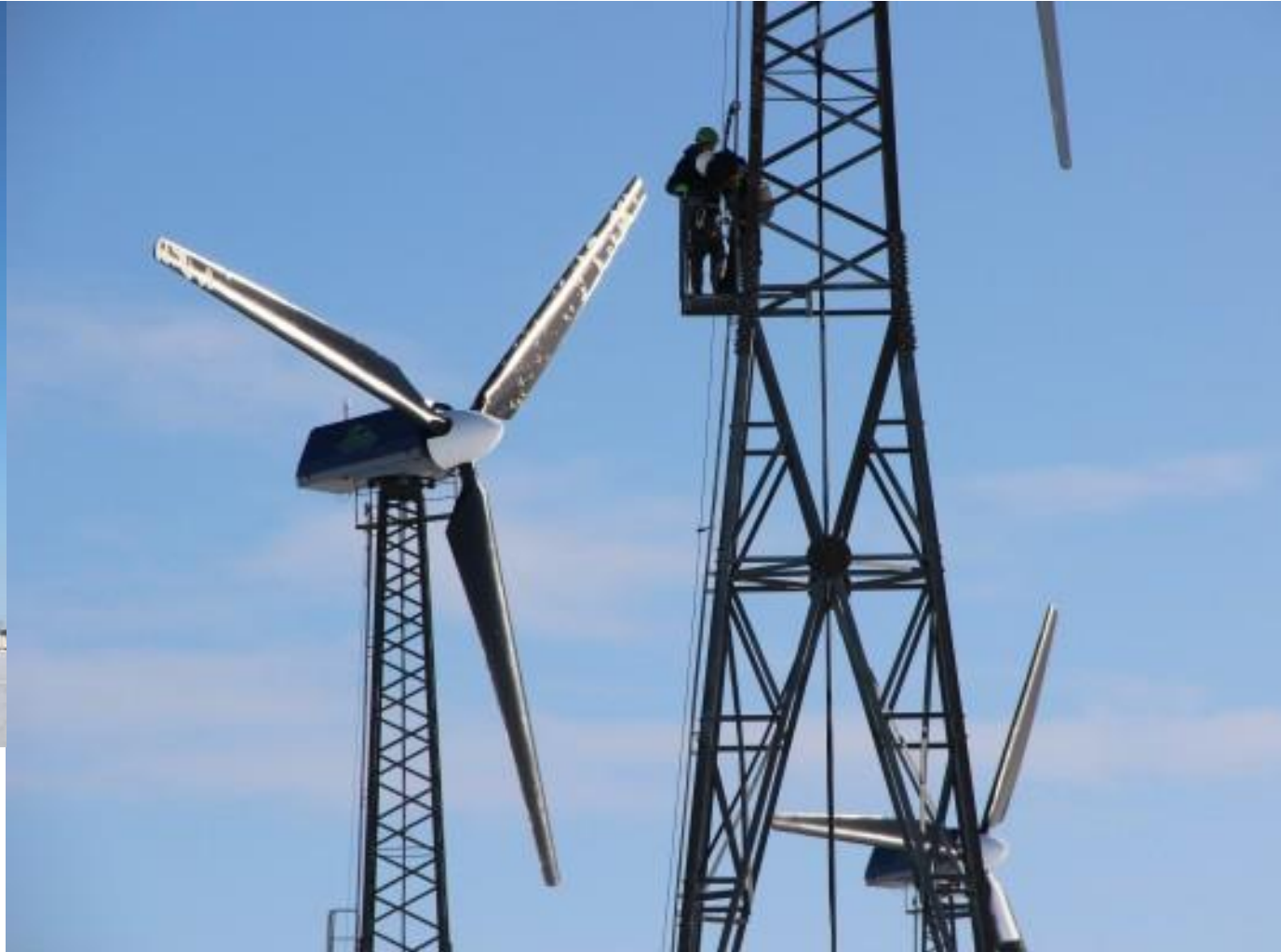
Patrick Boonstra of Intelligent Energy Systems, and Kwigillingok wind tech Benny Daniel check a turbine after a blizzard the night before. Photo: Rachel Waldholz/APRN
